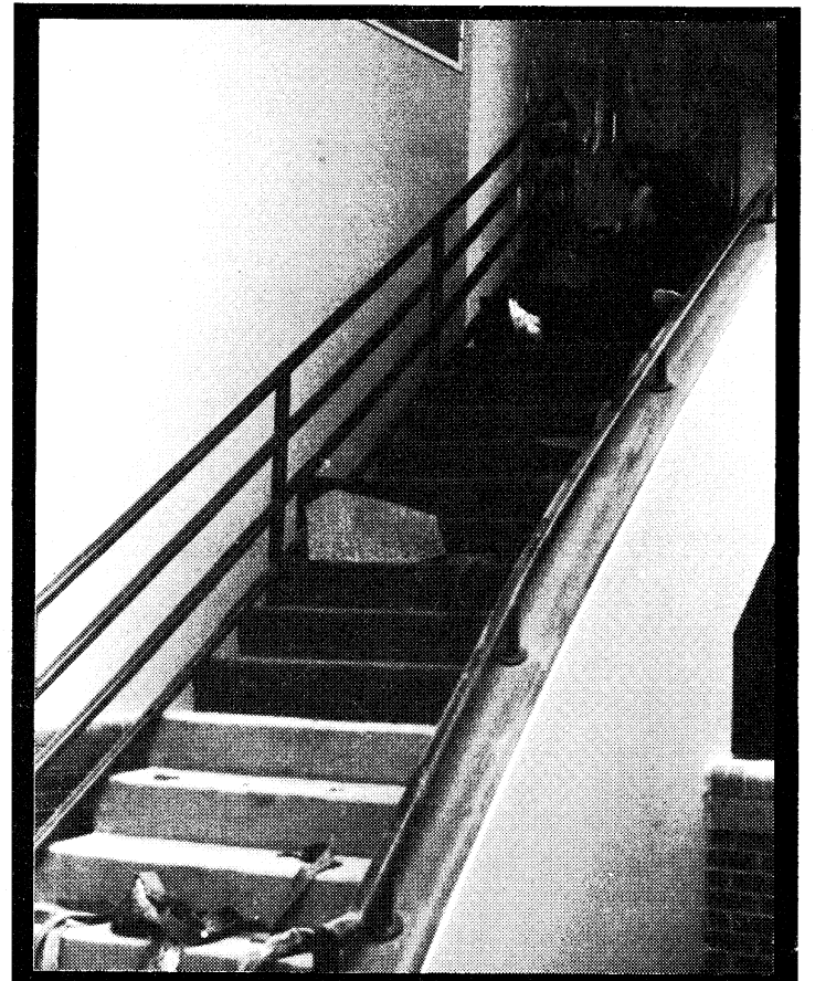
Construction workers install the carpet on stairs in the new Student Center. These stairs lead to the upper floor which houses the Ballroom, WGHR studios, main entrance and lobby, up-teengillion conference rooms, the Student Activities offices, Counseling Center offices, Trident missile assembly plant, and the four Southern Tech fusion reactors. - Photo by Jennifer Waller.
