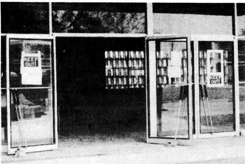
GUTTED GOATSHED: The Administration Building gets rid of poisonous asbestos while in the process of remodeling.
