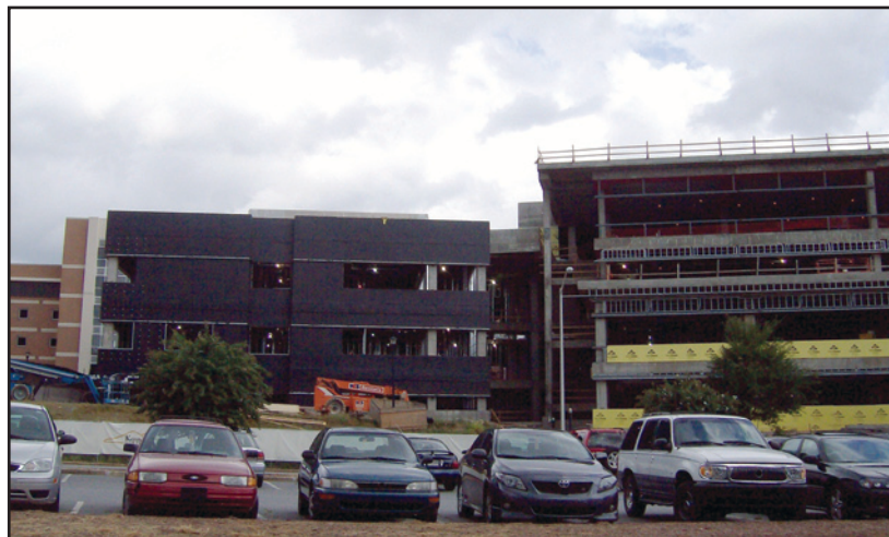
Karlee Gonzalez | The Sentinel The new Health Sciences Building, located between the Central Parking Deck and The Commons, is scheduled to open for classes in time for the fall 2010 semester.
